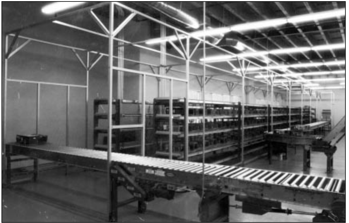
Computer Burn In Tunnel
